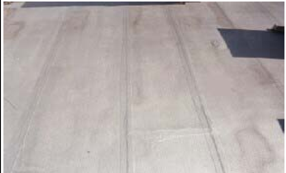
Two Years Old, Coated With Weather Barrier Moisture Cure Urethane. All Seams Were Taped For Additional Reinforcement . Weather Barrier OZ Catalyst Was Added To Resist Animal Fats.
